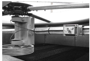
Figure 2: Typical 5550 installation on cooling tower fan support strut.
